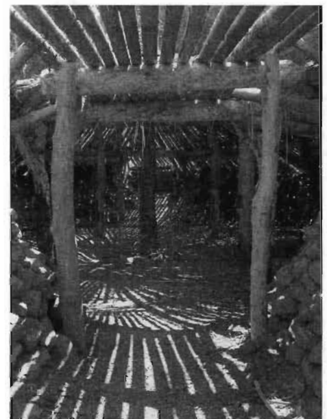
The round house under construction in 1983, seen from the low-roofed entrance way. Photo by Charles Kennard
