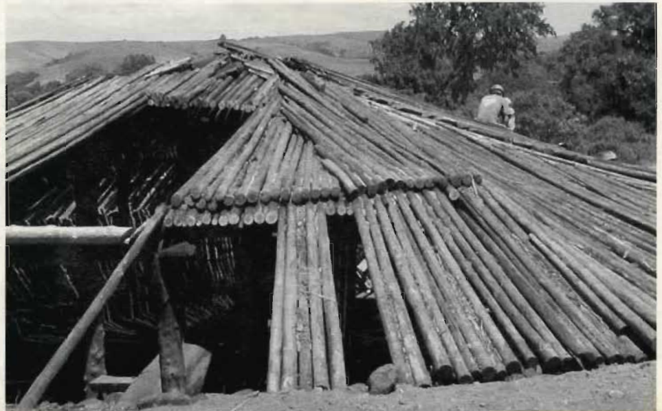
For the past year, Kule Loklo volunteers, tribal members and PRNS employees stripped bark and shaped Douglas fir poles with an eye on restoring the Roundhouse roof. This summer the roundhouse roof (shown here) was completed. photo courtesy of Gordon Bainbridge
