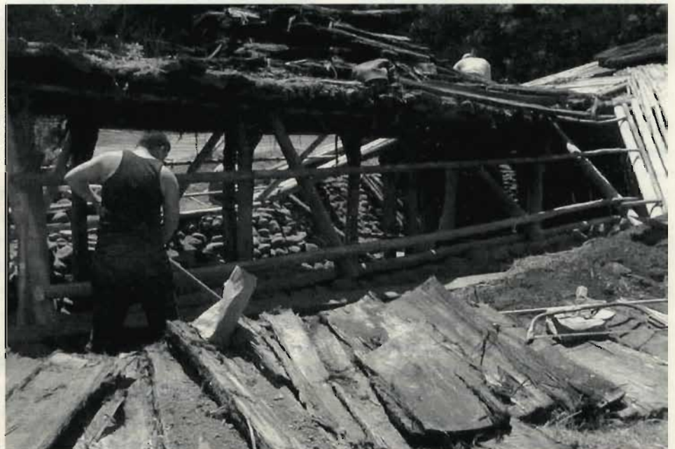
The entrance vestibule of the Roundhouse is reconstructed with new Douglas Fir poles and Redwood bark for siding. photo courtesy of Gordon Bainbridge
